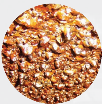
Varnish on reservoir ceiling ( Stalactites )
